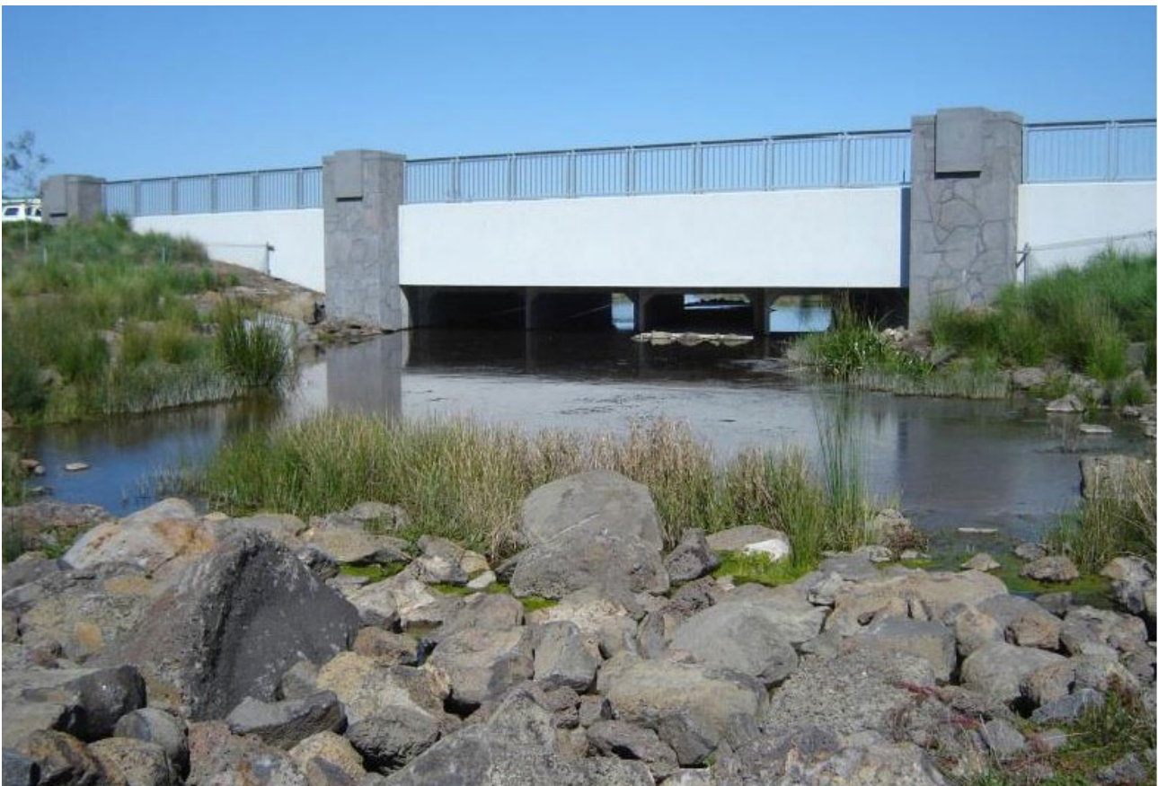
A 10 metre wide set of culverts, three of which are permanently inundated, provide passage for Growling Grass Frogs under a two-lane road over Edgars Creek. All images by Daniel Gilmore, Biosis Pty Ltd
